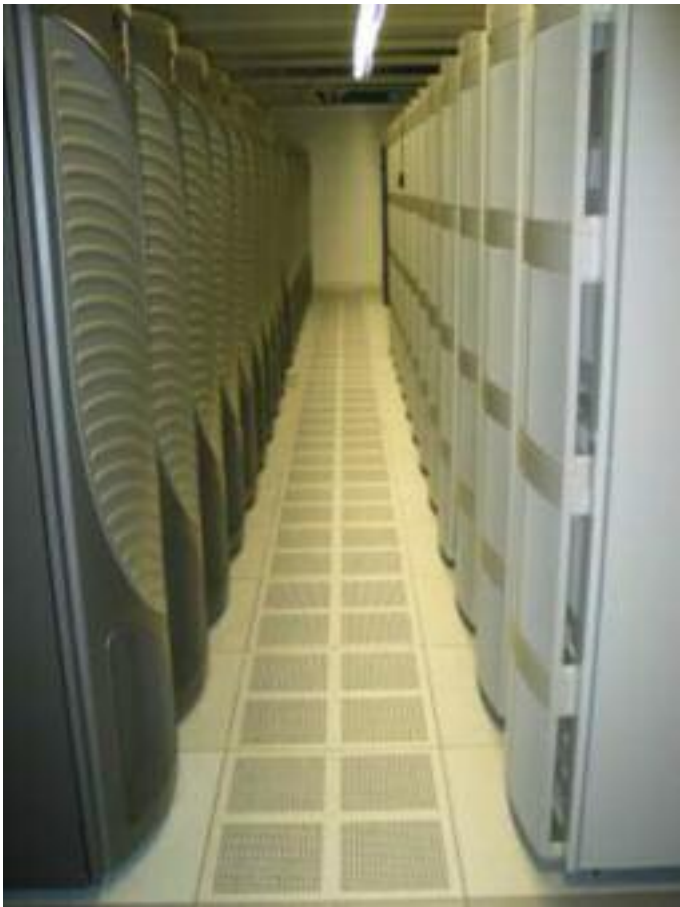
Four foot cold aisle but only one row of perforated floor tiles
