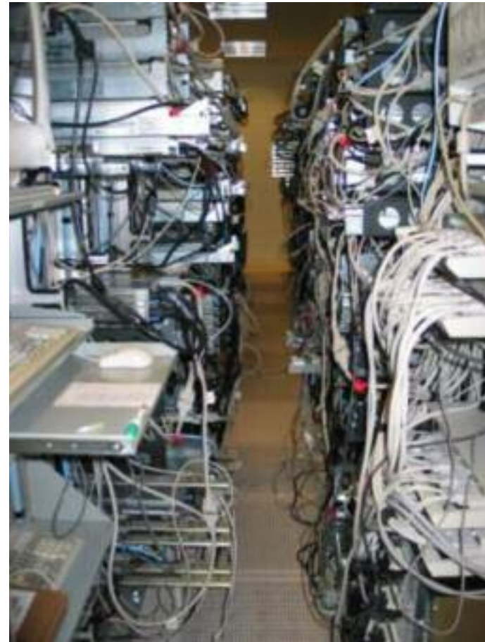
Poor cable mgmt blocks air flow through servers + perf tiles in the hot aisle
